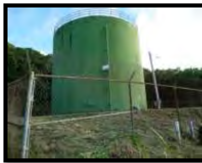
Photo 3.14-6. Carolinas Water Storage Tank (500,000 Gallon Tank)
